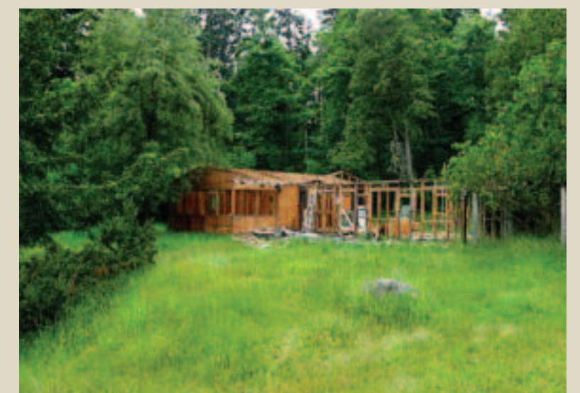
The Graham house during the deconstruction process. All building materials from this home will be reused or recycled.
